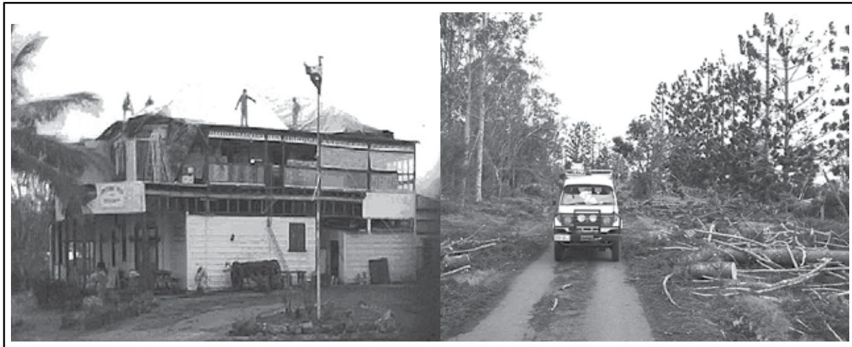
Pictured left: Local Kuranda SES member Paul McCorry helping tarp the roof of the Peeramon Pub after cyclone Larry
