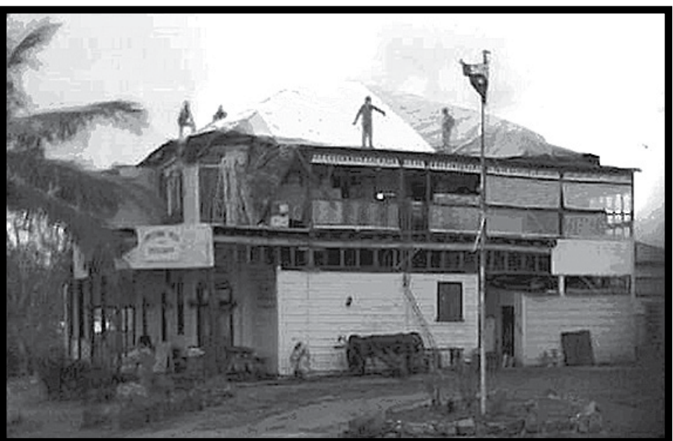
Local Kuranda SES member Paul McCorry helping tarp the roof of the Peeramon Pub after cyclone Larry.
