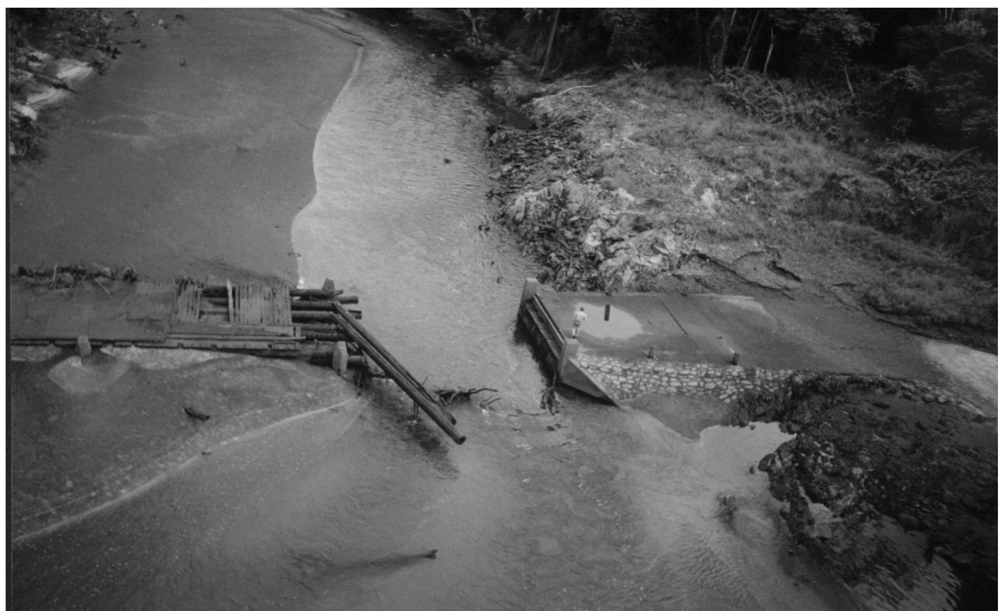
BARRON RIVER at lowest ebb. The lowering of the Barron River has exposed the old crossing,. Exposure of the river bed allowed the hydro power inlet to be checked and the sand which has accumulated to be assessed .
