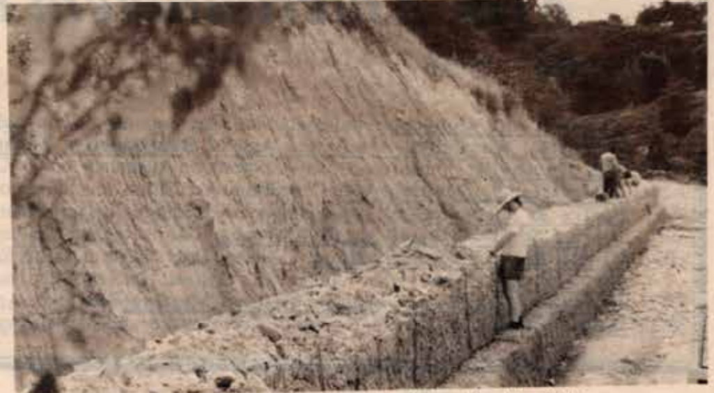
Soil retention at the Sports and Social Club. Well designed wall works behind the car parking area. Photo R.Dods
